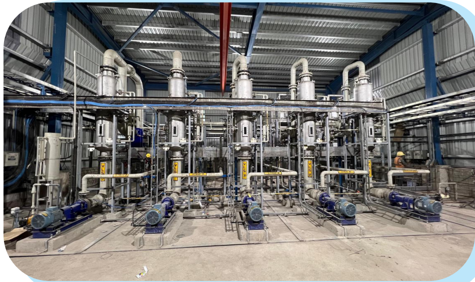
Waste Heat Evaporators
